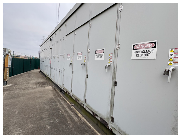
Traction Power Substation
